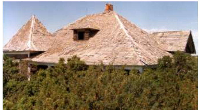
The derelict Dr. Malcolmson residence near Alliance, Alberta, photographed in 1992. This large house was cut into pieces, moved by rail, and reassembled on this farm. See our issue #8 for a few more photos of this house. Photo: Frank Slide Interpretive Centre
