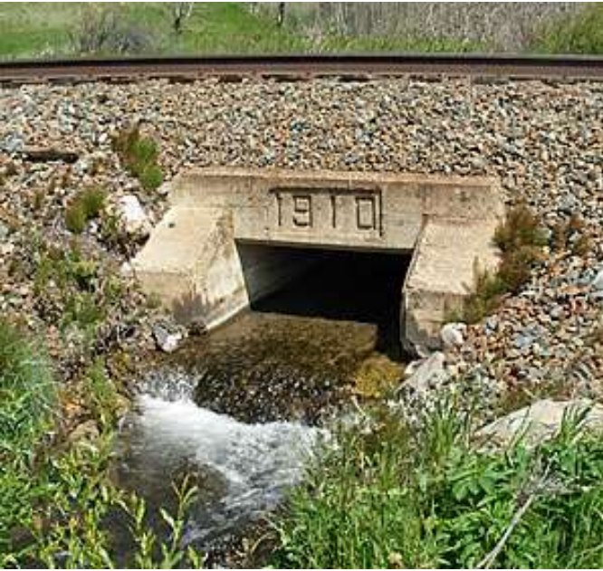
Concrete bridge just beyond the west end of Willow Drive. Photo: Ian McKenzie
