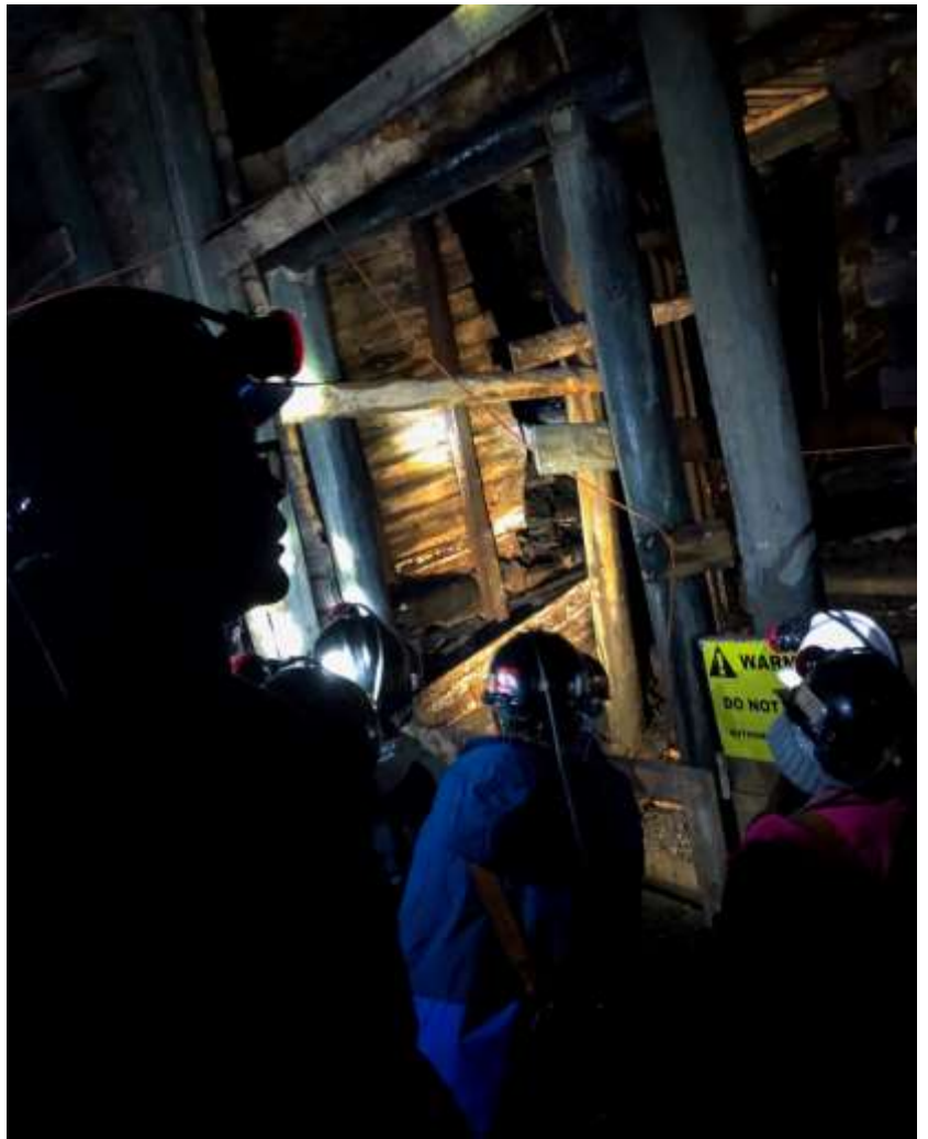
Staff observe a volunteer crew performing repairs to the "Man way" entrance tunnel.
