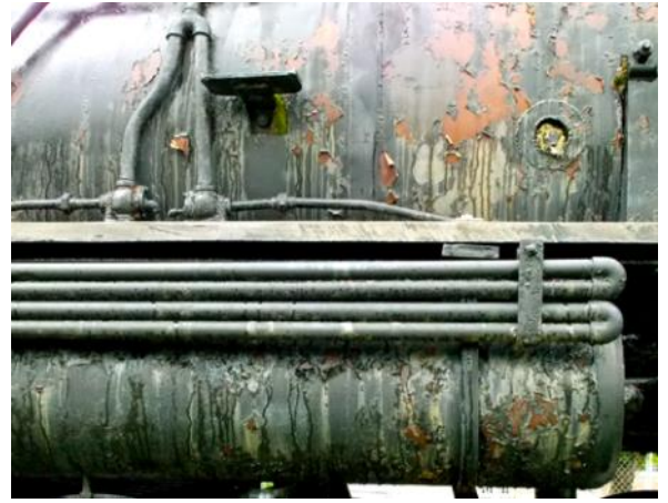
Detail of Old Maude rust, a result of exposure to the elements. Photo C. Allum
